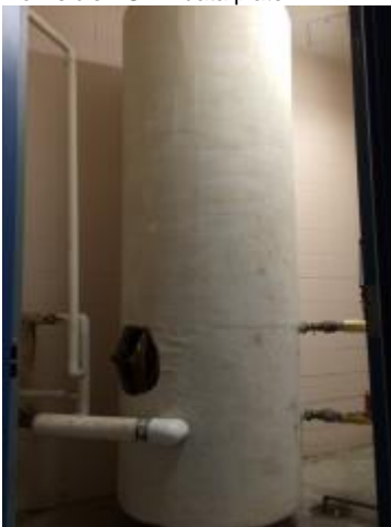
Photos No visible ASME data plate
