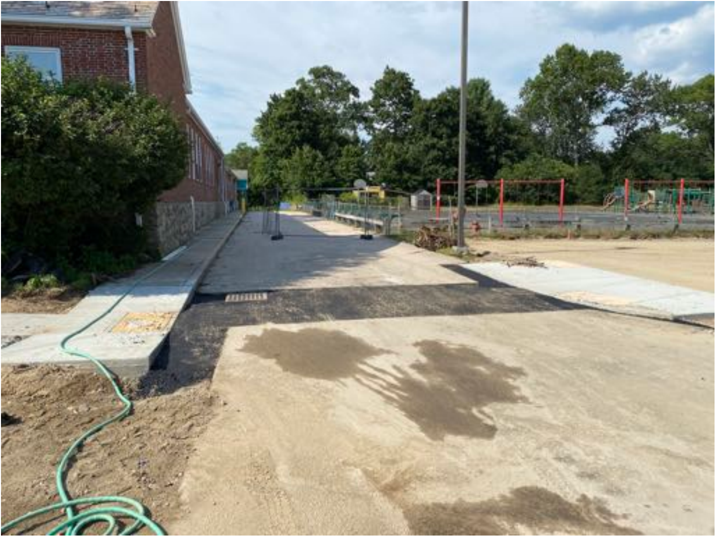
Asphalt patch at electrical conduit crossing.
